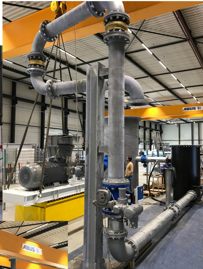
Closed test loop 250 OH type of pumps (API)
