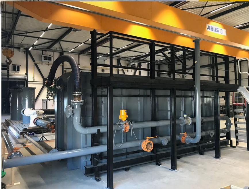
Open-pit testbed 200 VS type of pumps
